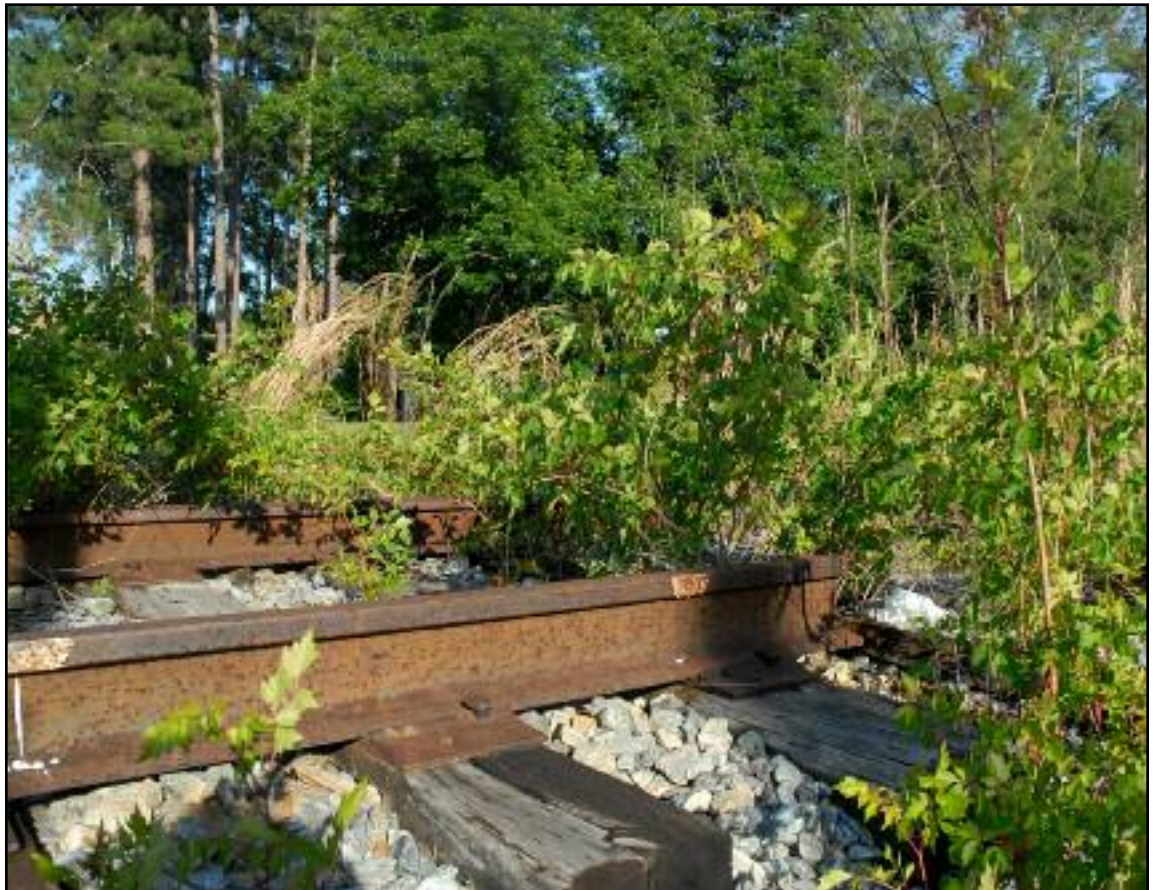
These are tracks that run behind Trinity Baptist Church. They literally just stop a few feet from the road they cross. Photo by Adelia Ladson
